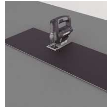
Step 5: Cut with a jig saw, hand saw, chop saw or guillotine cutter. Then snap the flooring - similar to scoring and snapping drywall.
